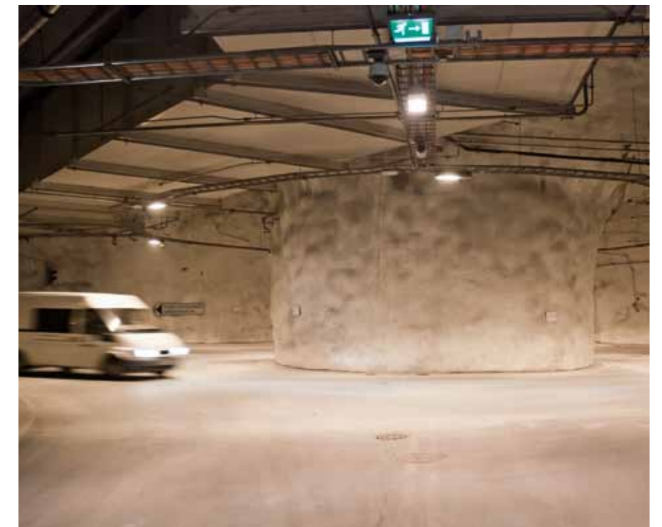
A rarity in tunnels, HI-FOG® protects all four KeHu roundabouts
