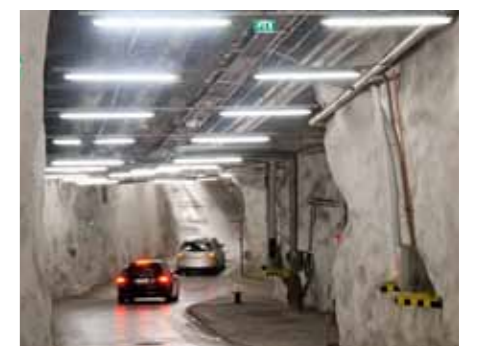
HI-FOG® offered a fast and cost efficient solution to replace the old ineffective sprinkler system in the Kluuvi tunnel.
